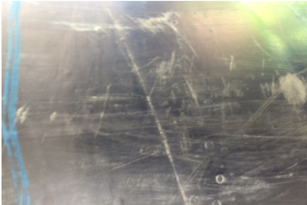
Close up picture of station 565+85 at the 4:00/4:30 location. No coating damage or dent detected
