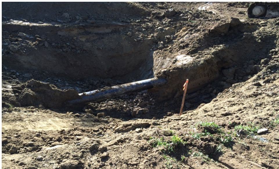
Exposed pipe section at station 565+85. Moved stake into area to show location of possible dent.
