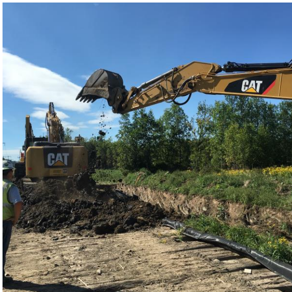
Photograph 4: Working off timber mats in stream buffer as excavation approaches stream 2012-SC-RS-5.
