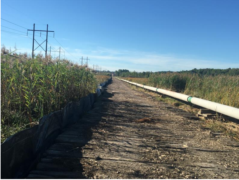
Photograph 7: New Haven Swamp viewed from the north facing south. No excavation to date.
