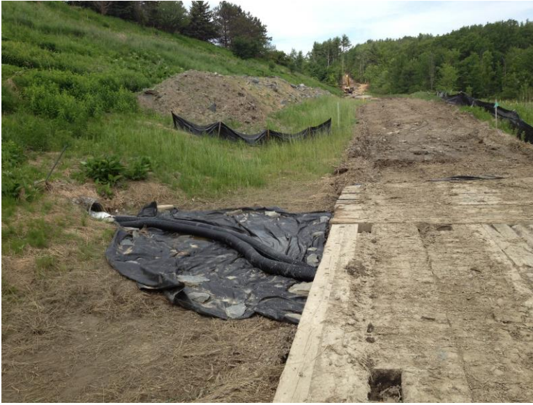
Photograph 3: Wetland mats continue to be maintained through resource areas as work continues around Indian Brook.
