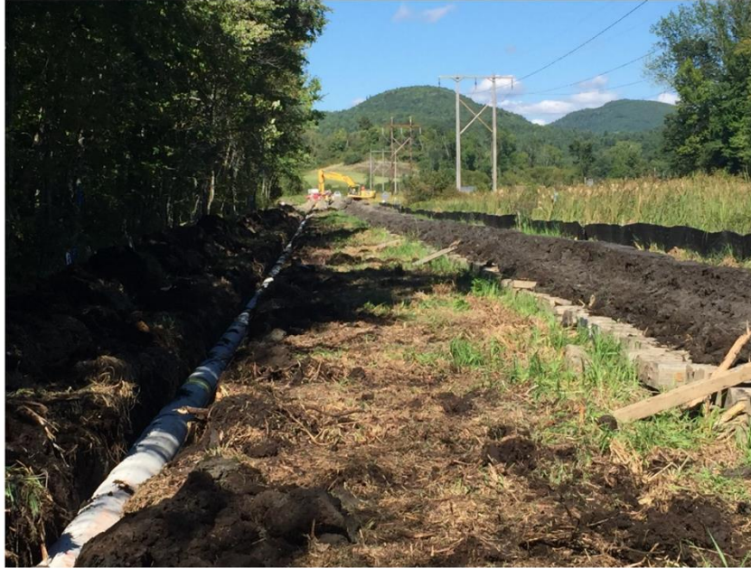
Photograph 4: Station 1649+00; trenching and lowering in the pipe through Clay Plains. Topsoil and subsoil are segregated and placed on timber mats. Photograph taken looking north.
