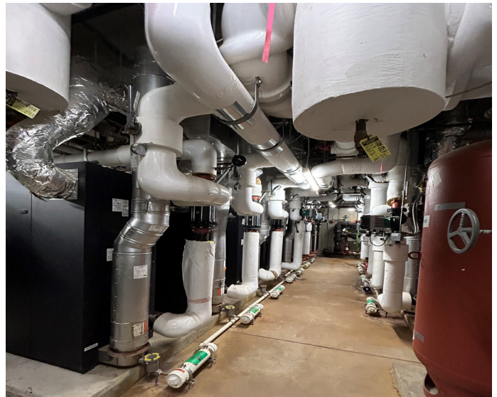
A look inside Jay Peak's boiler room, where a newly upgraded electric boiler system is helping to cut the resort's carbon emissions.
