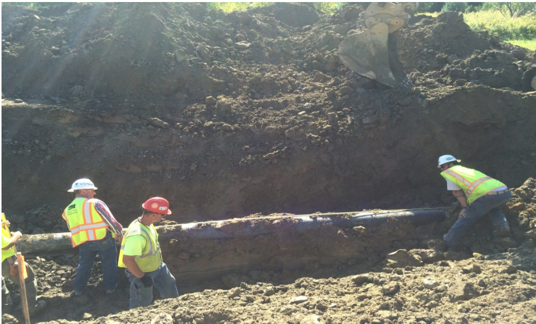
Measurement of 17' from weld 0193 to possible dent to confirm location.
