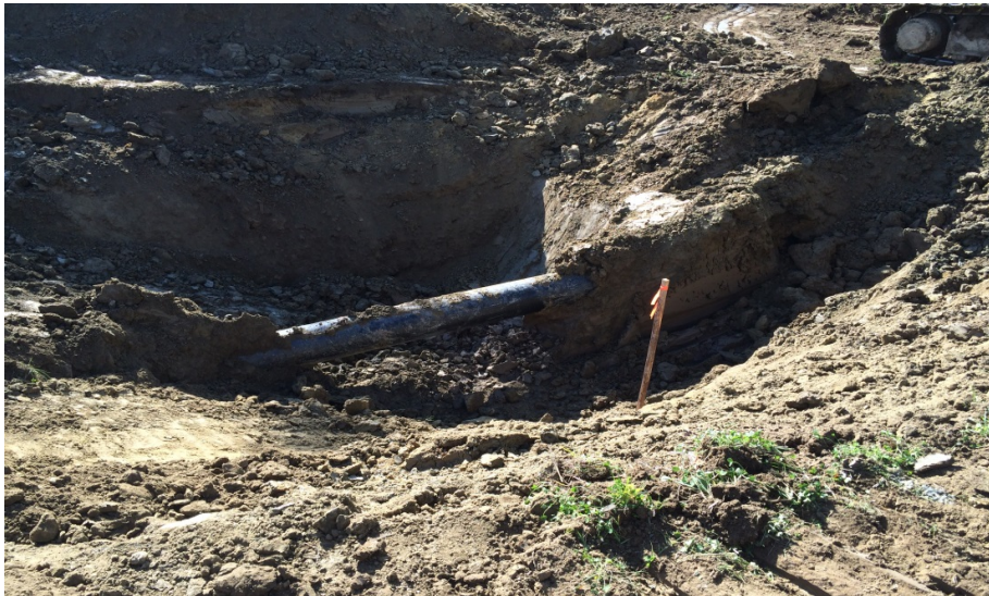
Exposed pipe section at station 565+85. Moved stake into area to show location of possible dent.
