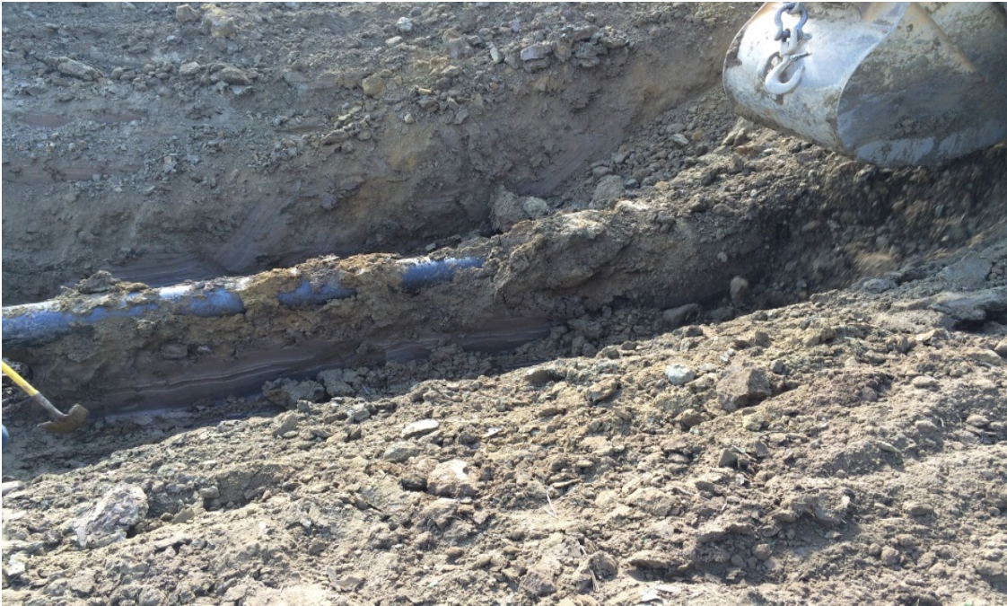
Exposing more pipe to weld 0193. No rocks detected just clumps of clay and clay topsoil mix.
