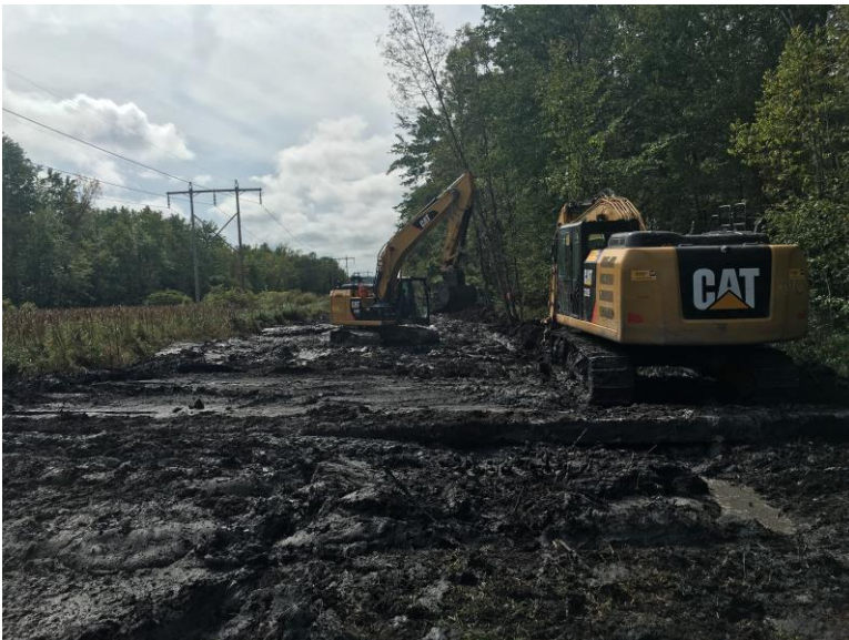
Photograph 6: Conditions were extremely challenging in the Red Maple/Green Ash Swamp. Crews continued to work off timber mats and managed to keep materials within the work limits to the best of their ability.
