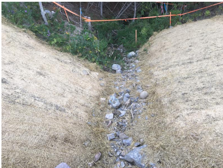
Photograph 1: Stream 2012-TB/SC-RS-3 crossing between Hollow Road and Post Road in Monkton is complete and restored. Stream is located at Station 1406+00. Stream was dry at the time of the crossing and remains dry as of the date of this report.
