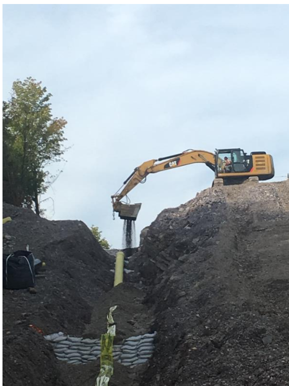
Photograph 2: Backfill between Hollow Road and Post Road in Monkton. Trench breaker shown in foreground. Utilizing shaker bucket to sift out material being placed in the backfill.
