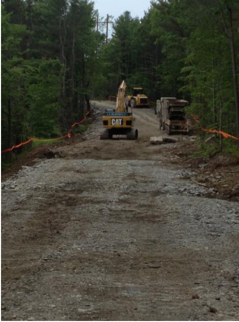
Photograph 1: J.A. McDonald, Inc. setting up their rock crushing plant to process the blasted material so that it's suitable for general pipe backfill. Plant is setup within the ROW off of 289.
