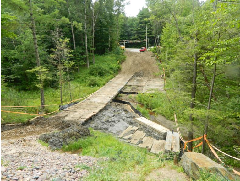
Photograph 1: Michels Pipeline Construction installing timber mats and access to Redmond Brook stream crossing. Matting also being installed in adjacent wetland 2012-CM-134.
